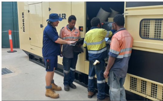
Clarke Energy Australia
