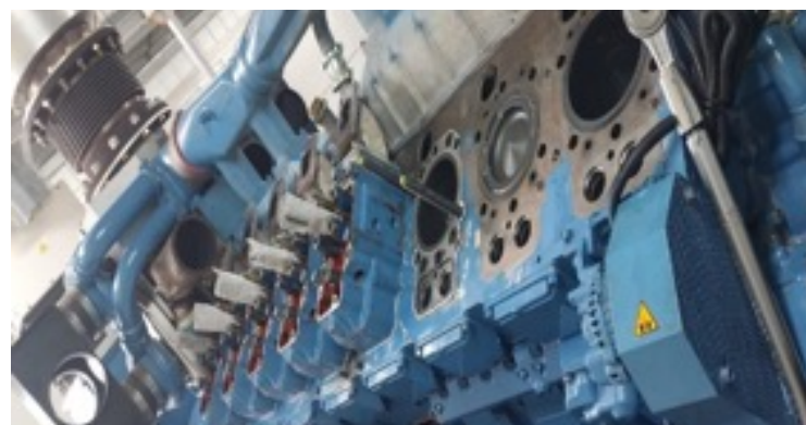
Open engine ready for maintenance. All injectors and head cylinders have been removed to control their good running (fuel pressure tests, fuel and gaz valves, rocker arms, etc.)
