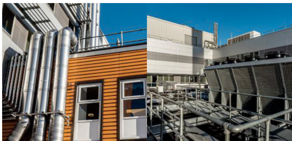
The newly installed pipework and flue system, which was designed and installed by WB Power Services.
