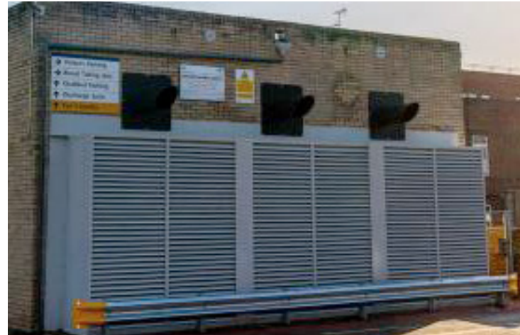
The newly installed outlet attenuators for generators 4, 5 and 6.
