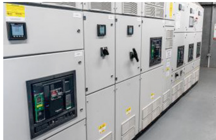
Newly installed T1250 KOHLER-SDMO generators and switchgear in place within the plant room
