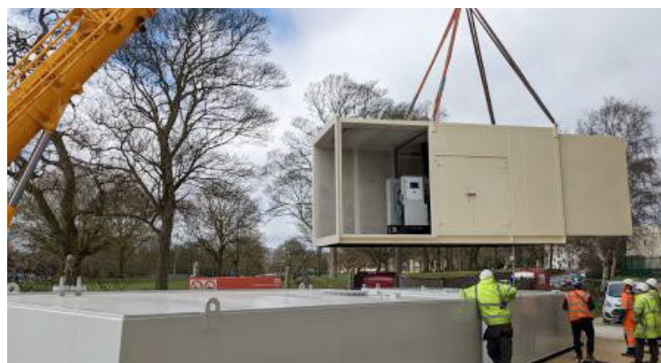
As part of the installation, the incumbent generators were removed, refurbished and re-installed by WB Power Services
